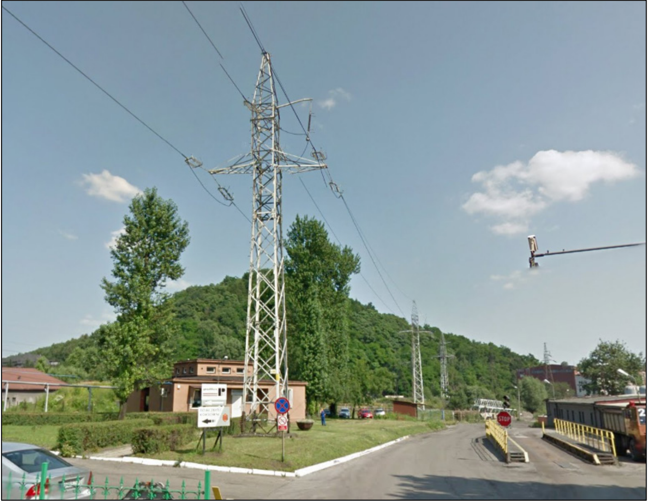
Figure 28: 110kV Power Line into Debiensko
