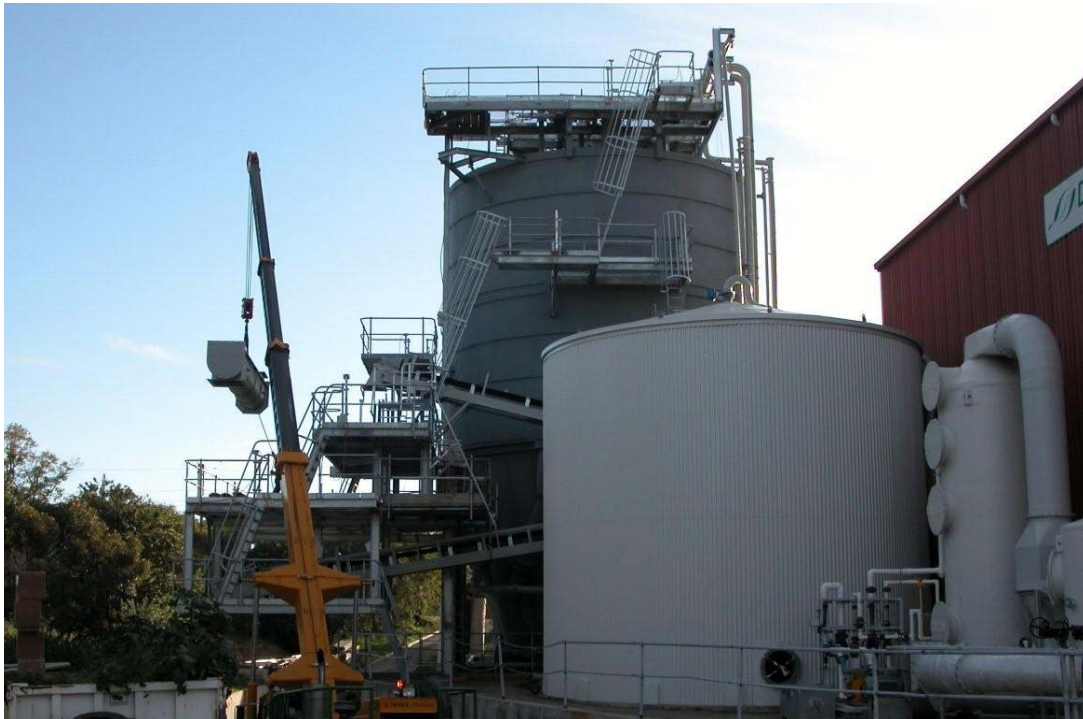
1 DiCOM bioconversion vessel with water tank and odour management system in foreground
