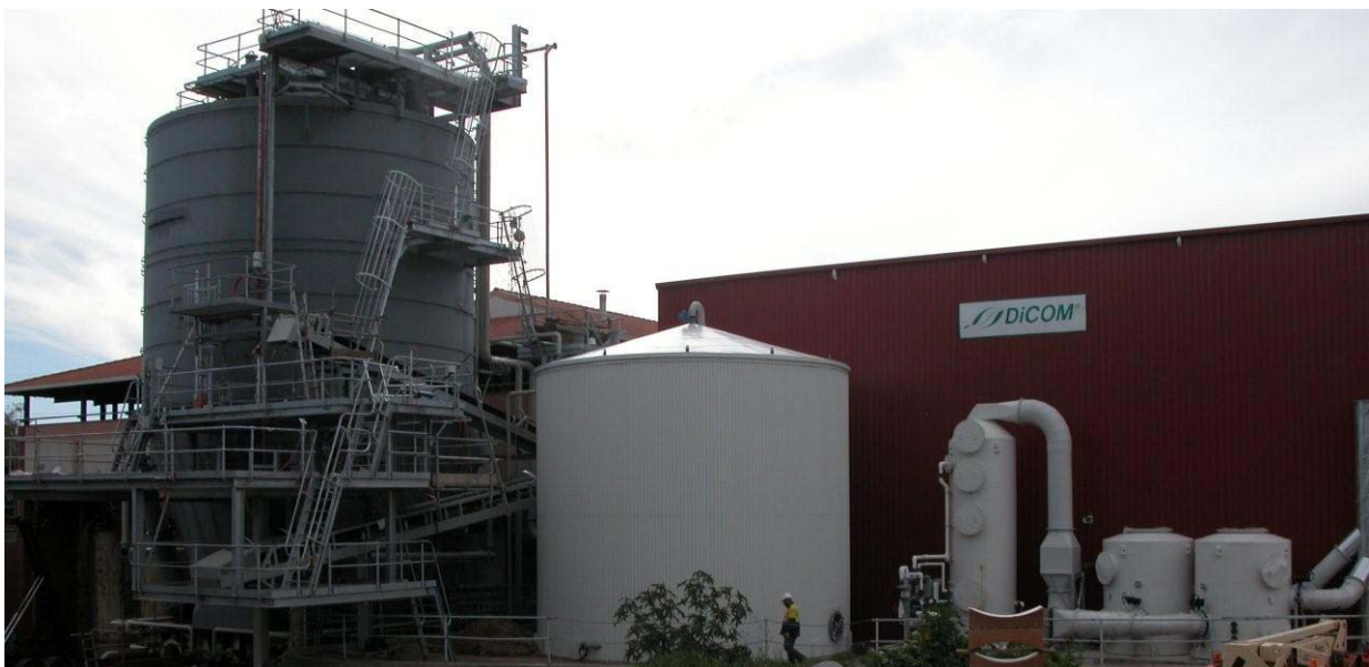
2 DiCOM bioconversion vessel with water tank and odour management system
