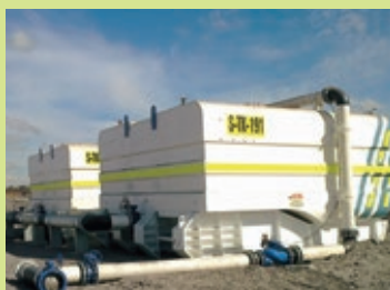
In-pit water tanks.
