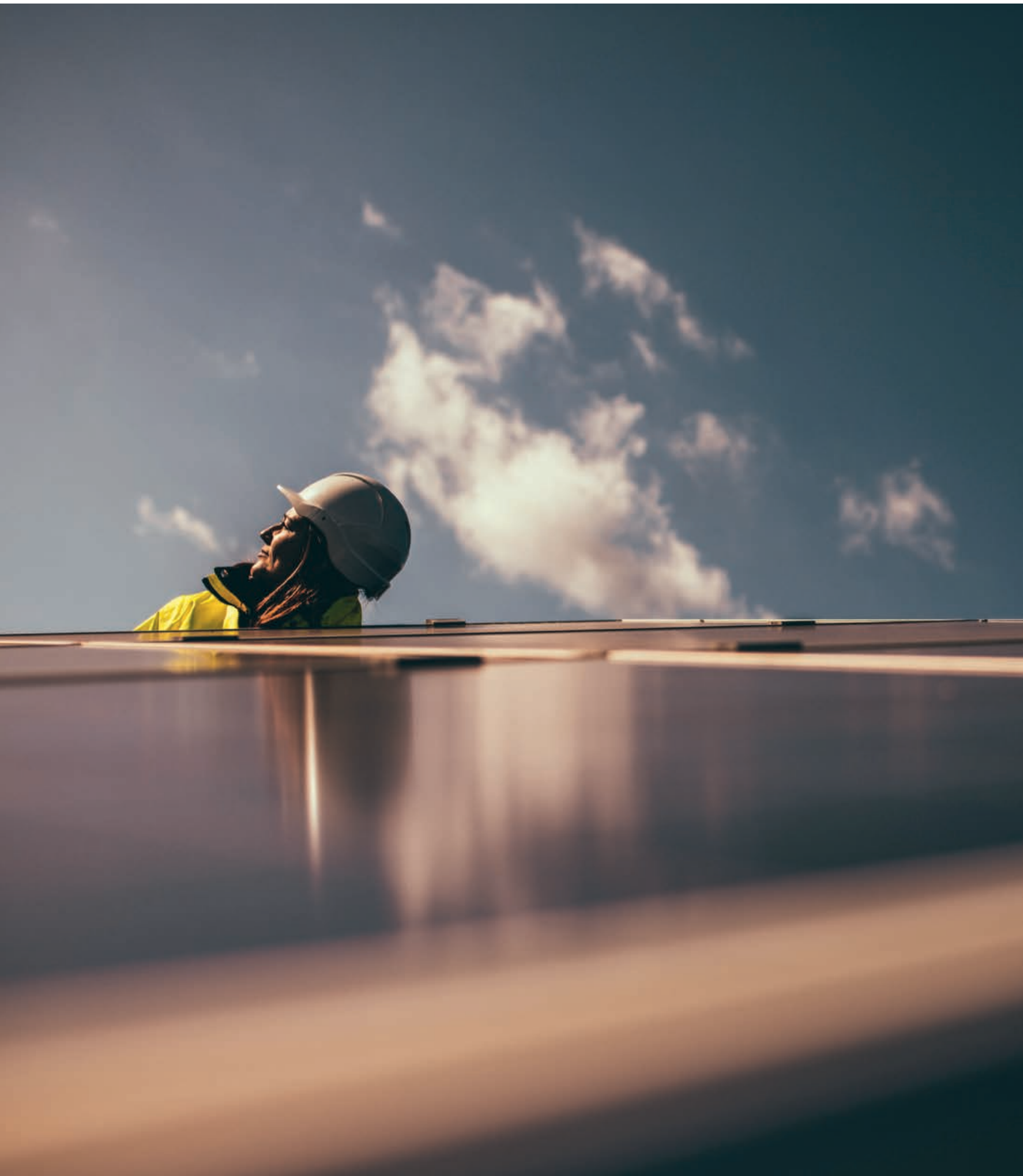
Photo by Arlindo Camacho, Photovoltaic installation - Portugal, 2018
