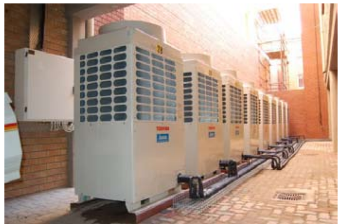
The picture shows the air-conditioning system which Metraclark has delivered to the Road and Transport Department in the Limpopo province in South Africa.
