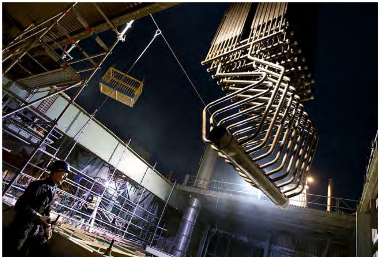
Modernisation of the recovery boiler at the Smurfit Kappa Kraftliner Piteå Ab paper and pulp mill will improve the availability and efficiency of the mill and increase its power generation capacity.
