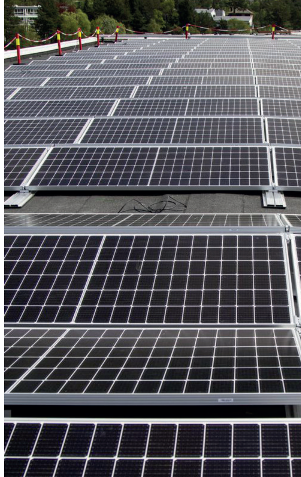
Solar panels at the roof of our headquarters in Fyllingsdalen.
