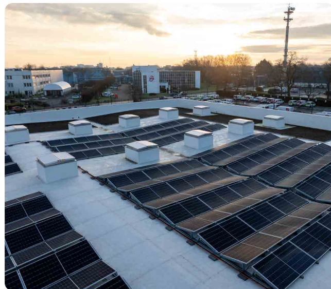
bpost NV/SA mail center Solar panels
