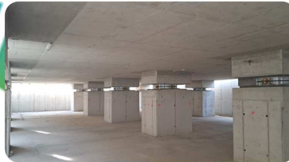
Sulmona Compressor Station – Seismic isolation devices in the underground technical room of the main building
