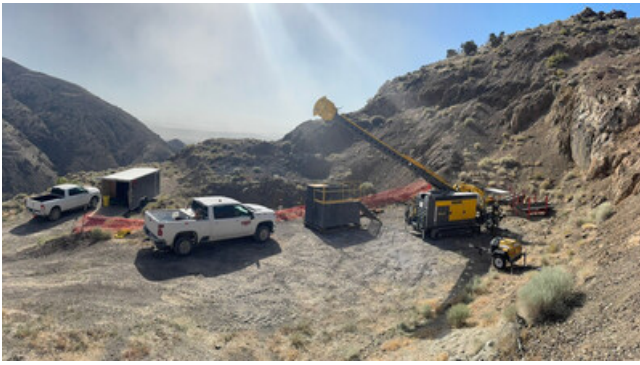
Figure 1: Drill Rig set to commence drilling FCG25-29 in the historic Colorado Pit (CNW Group/Getchell Gold Corp.)
