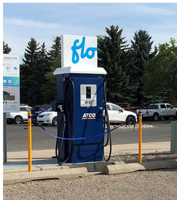
EV charging station, Lethbridge, Alberta
