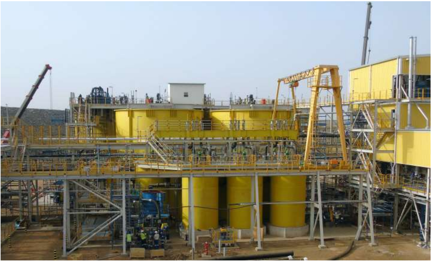
CIP and Leaching Areas
