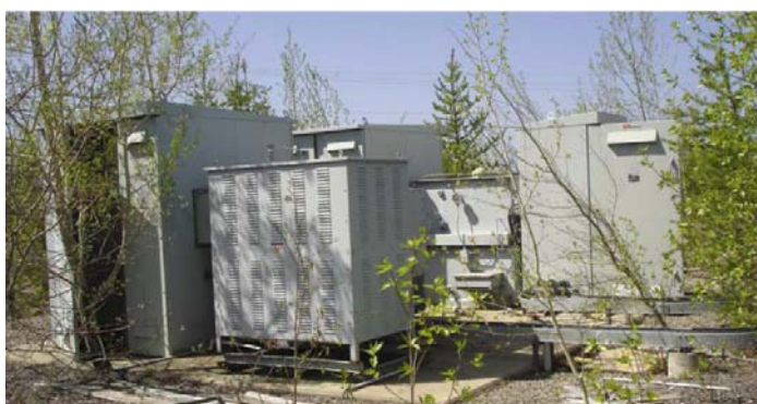
Figure 4-3. Substation General view of sub-station – remarkably good condition.
