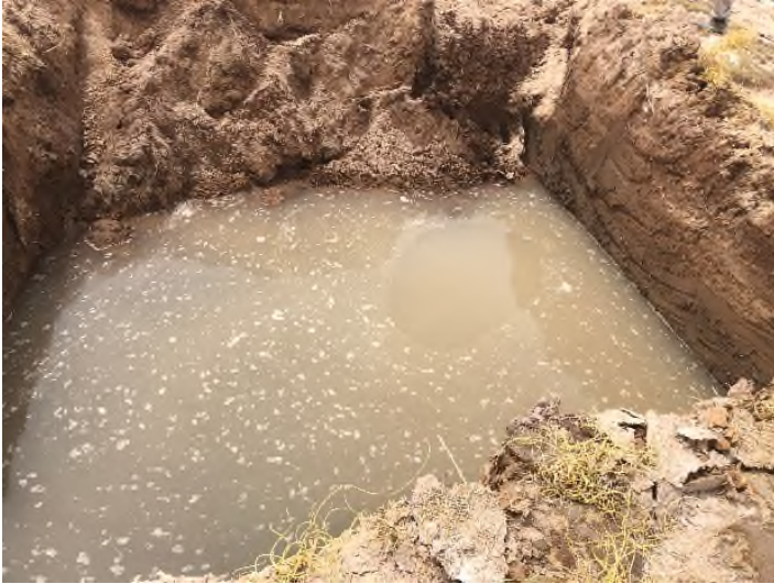
Fig 1 shows the significant amount of brine that flowed into the 5m x 4m x 4m pit some 36,000 litres within 18 hours
