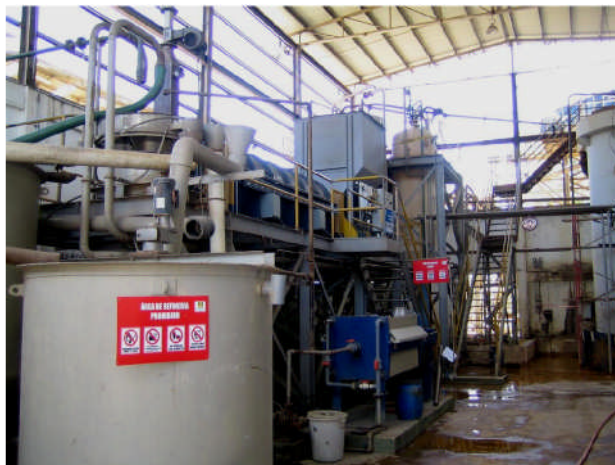
Figure 11 Carbon Column Systems
