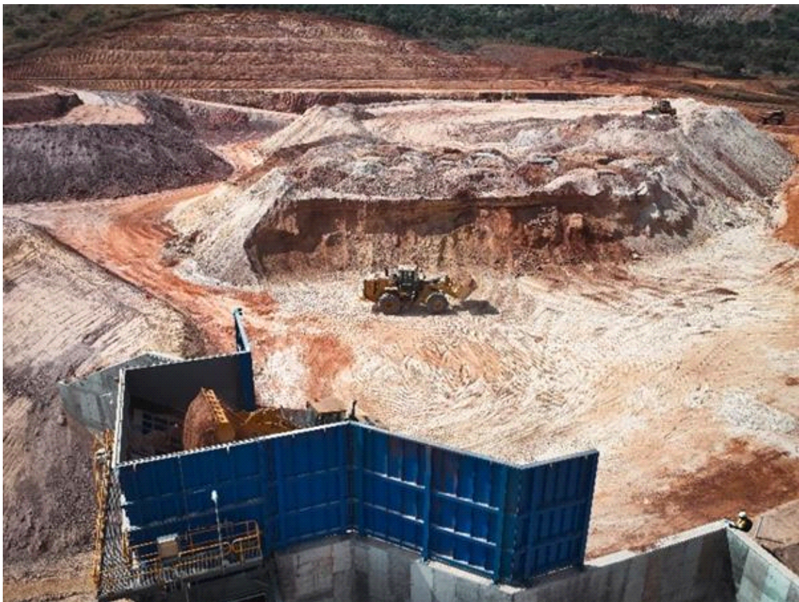
Figure 4: Ore Feed to Saprolite Crusher
