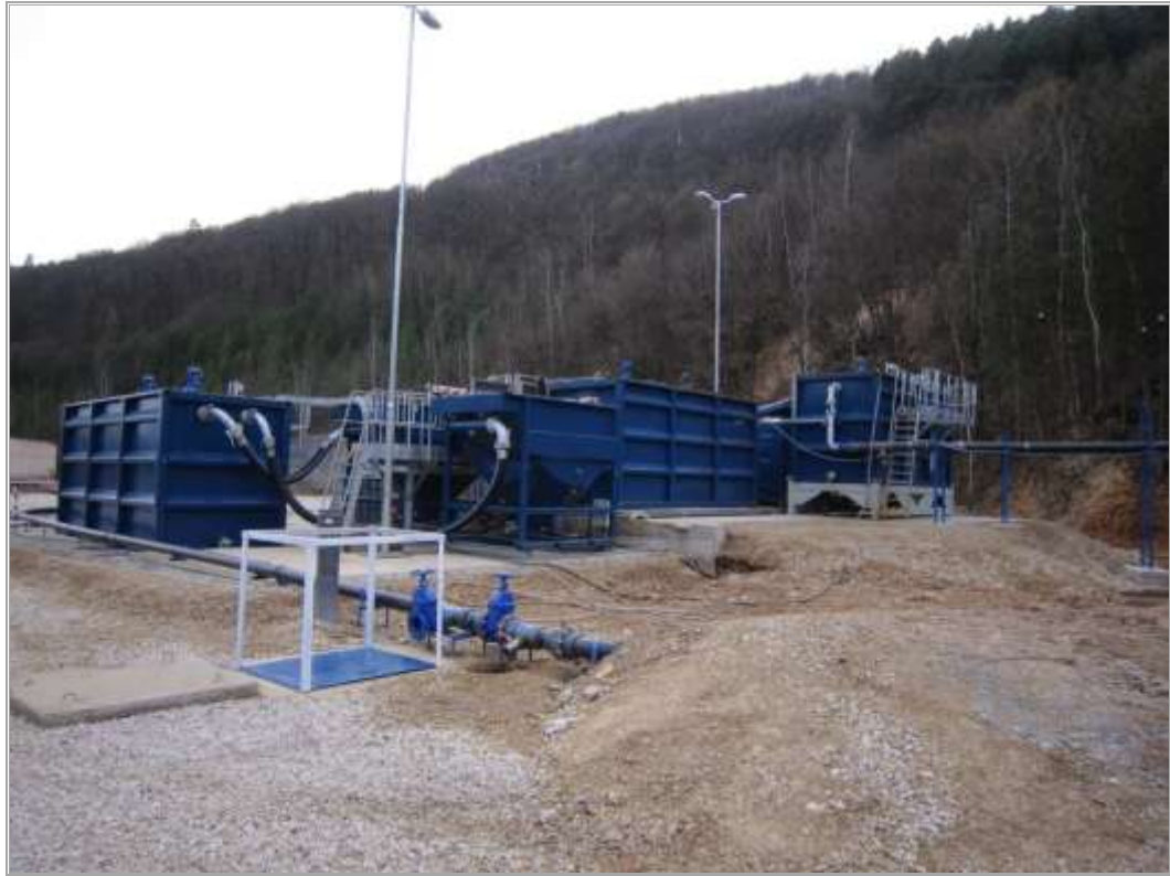
Figure 20-2: Strieborná Project Water Treatment Facility
