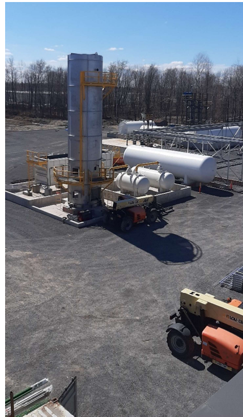
Ground flare, immersion coil and oil fractionation
