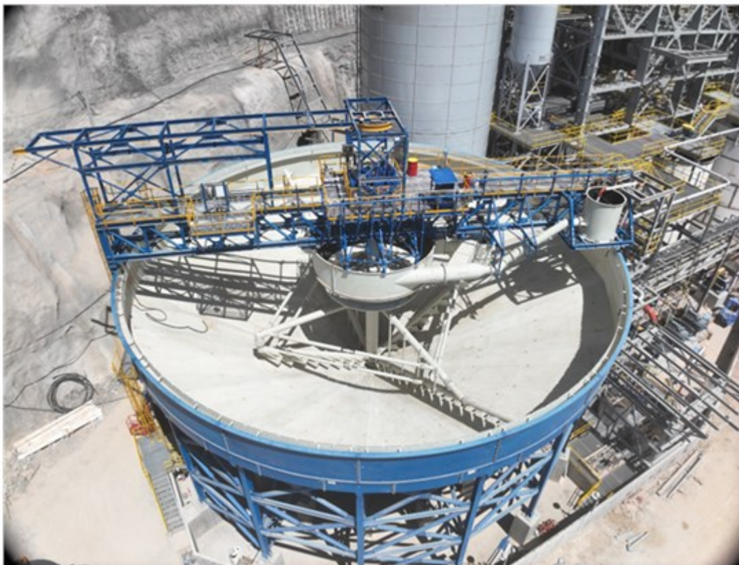
Figure 4: Paste plant thickener ready for water testing.
