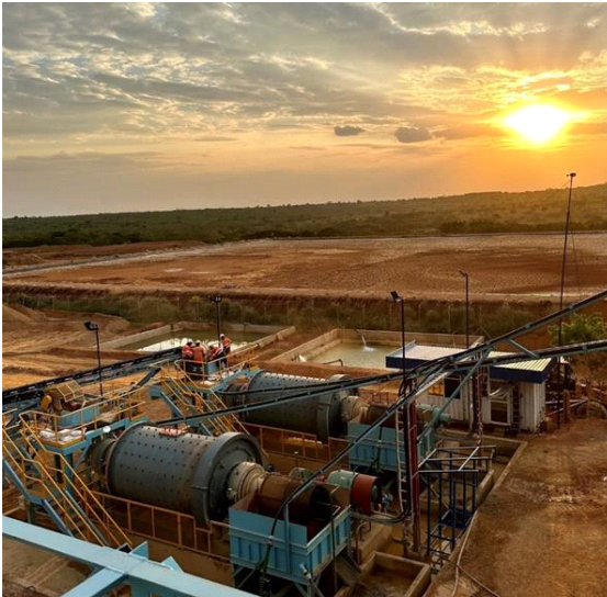
Figure 1. Buckreef Gold Expanded 1,000 tpd Processing Plant in Q1 2023, showing installation of two new 360 tpd ball mills.
