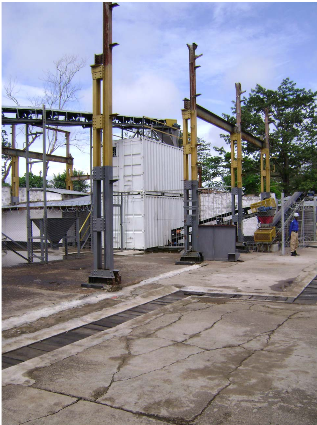
Photo 14 Final Recovery Unit, Kono Plant
