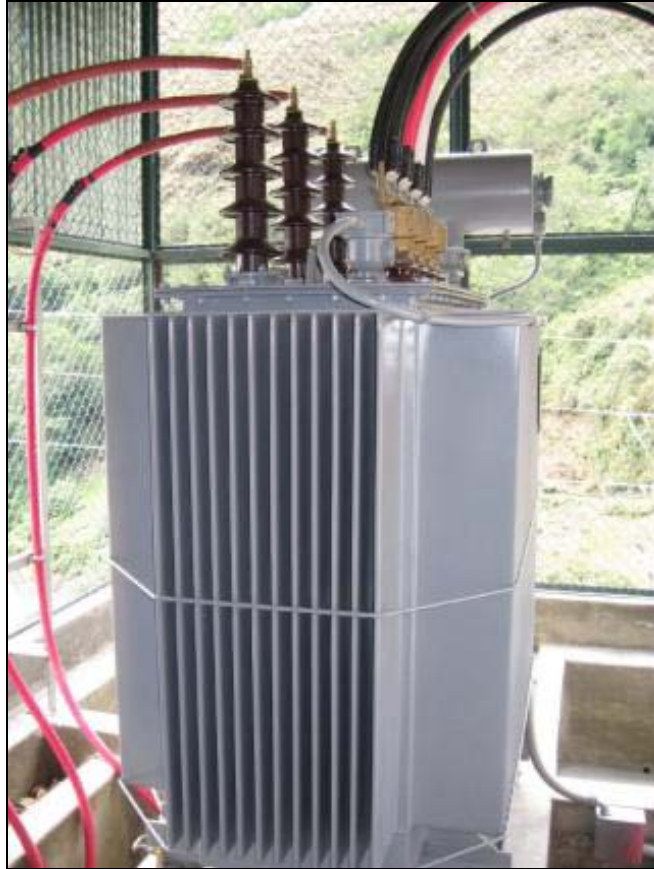
Photo 4: Power transformer in hydroelectric plant.
