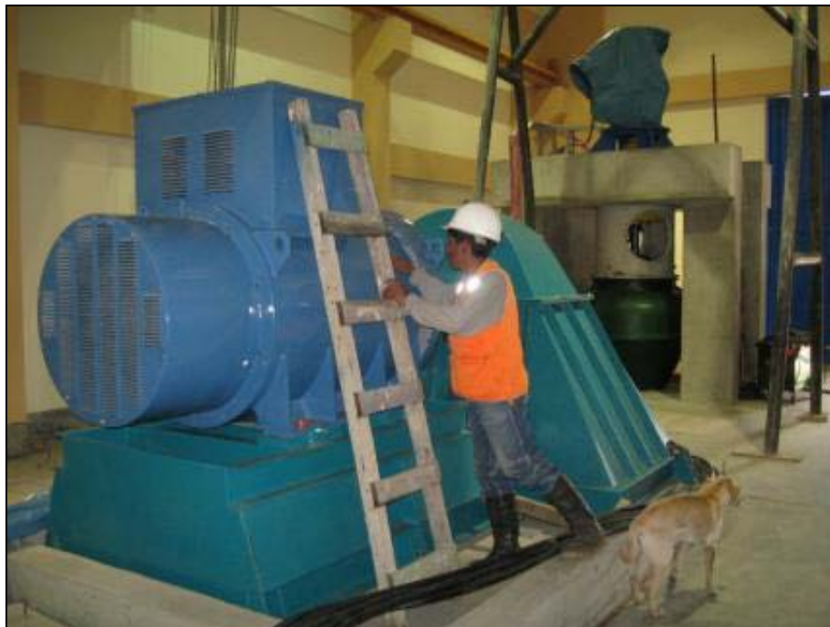
Photo 5: 700 MW generator in hydroelectric plant.
