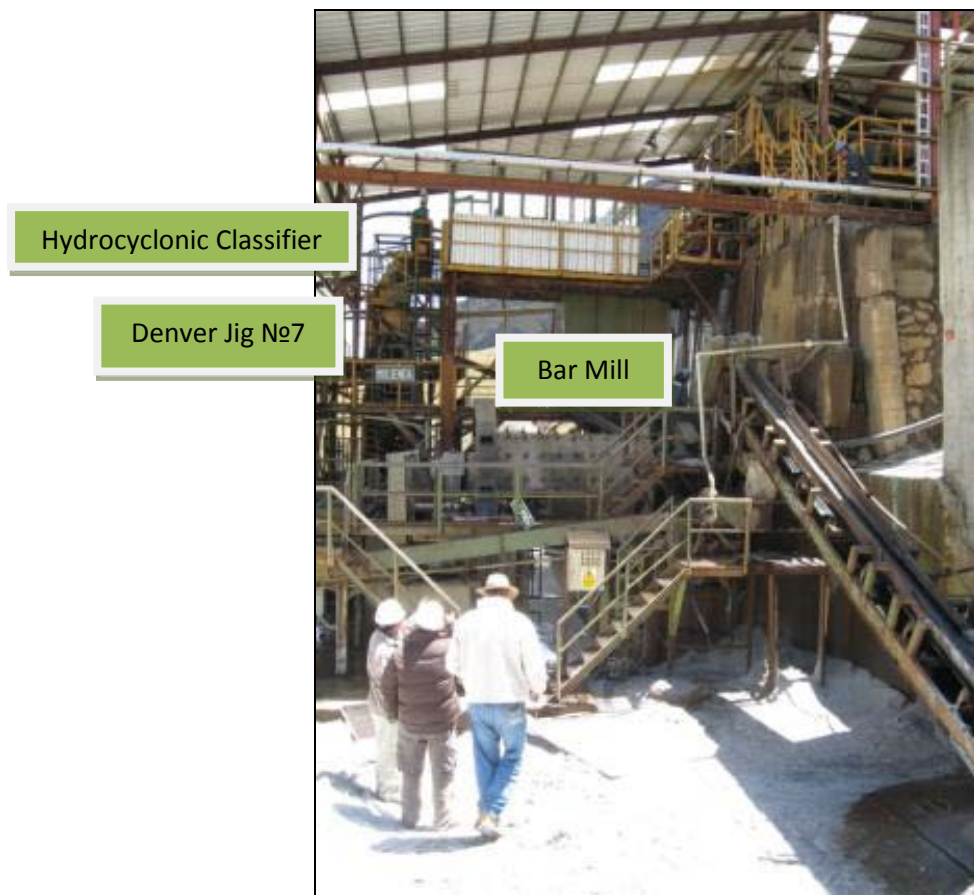
Photo 12: Bar mill, Denver Jig №7 and Hydrocyclonic Classifier
