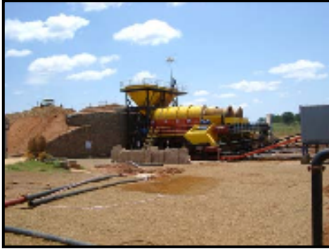
Scrubbers feeding new pan plant circuits
