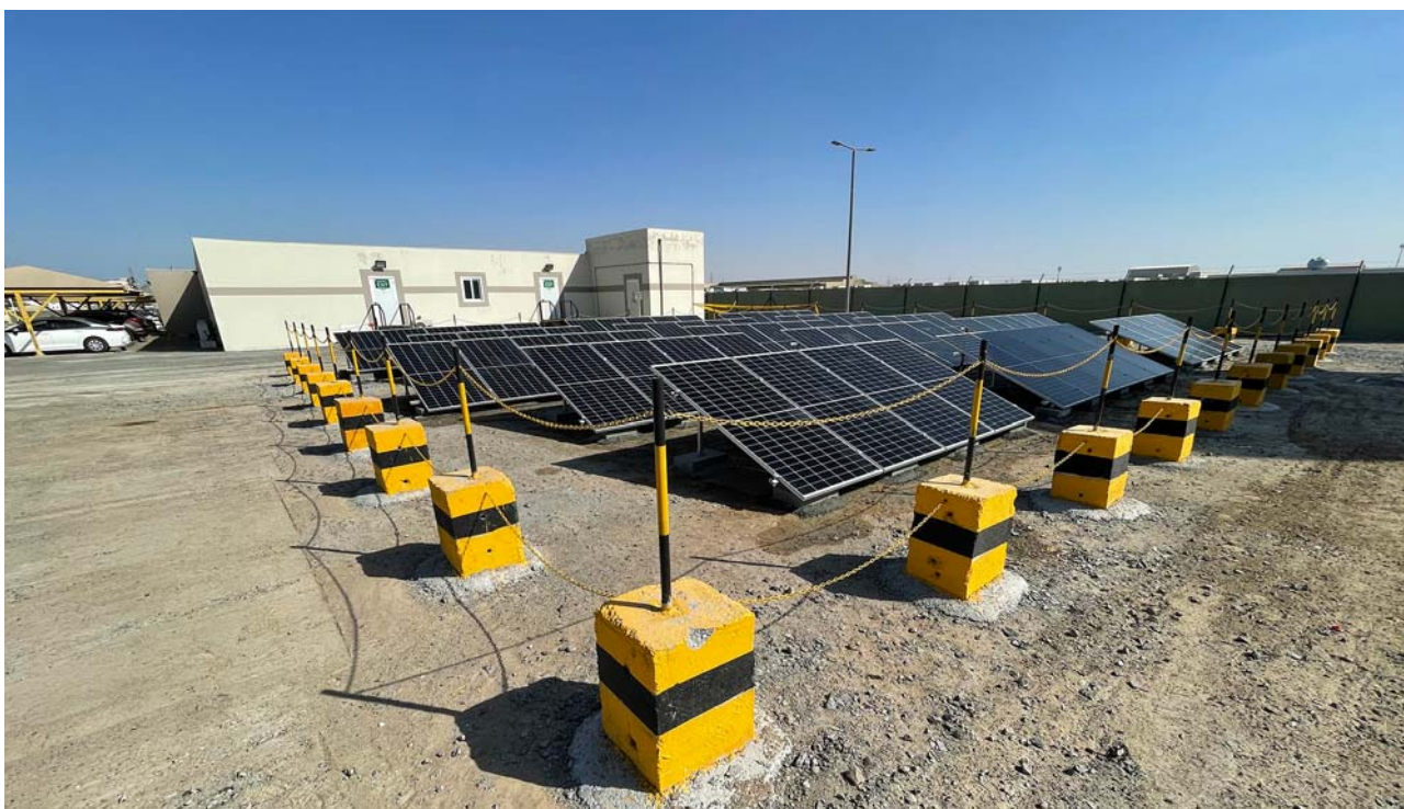
■ Hamriyah logistic base.
