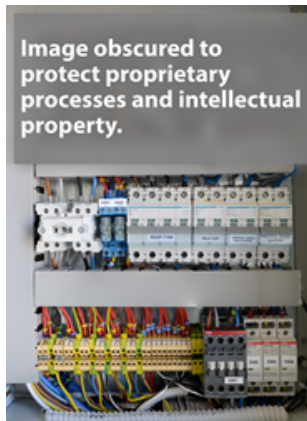
Climate Controls Panel
