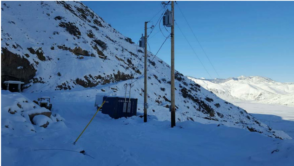
Figure 1: Electrical Power Connection at the Bayhorse Silver Mine
