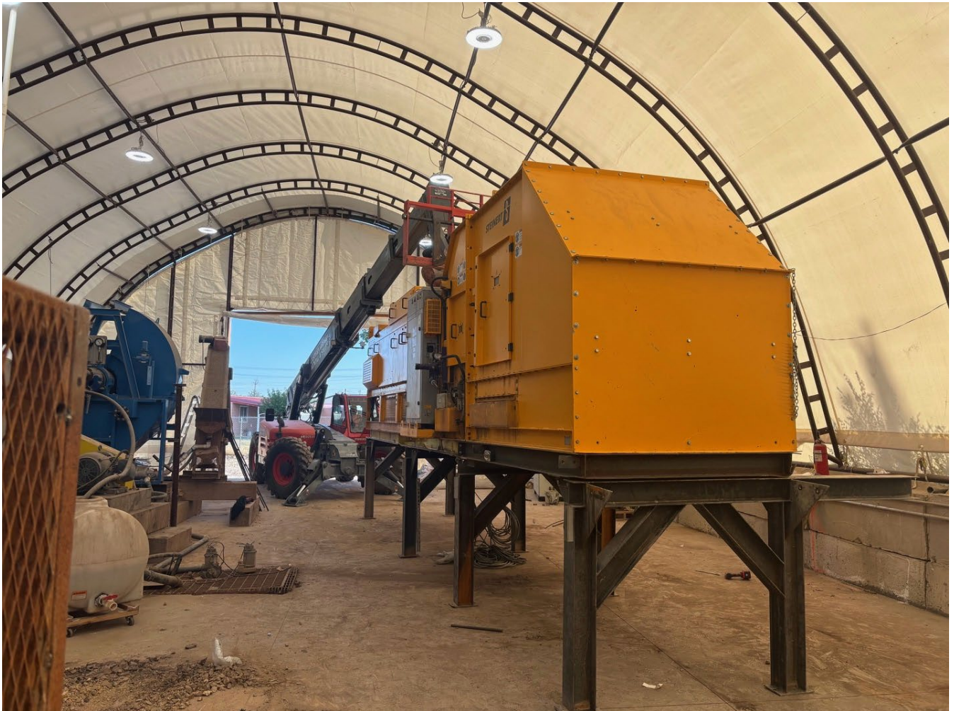
Figure 1. Company's Steinert Ore-Sorter installation at the Bayhorse Mill, Payette, Idaho
