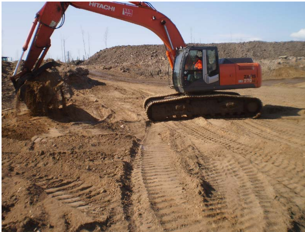
Photo 1 Location of TH321 within access road material excavation pit 2 (middle of pit along south end)
