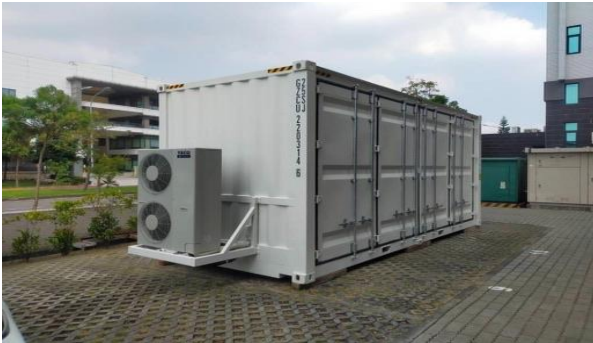
40 foot Containers used for Large Battery Storage Systems, external cooling for climate
