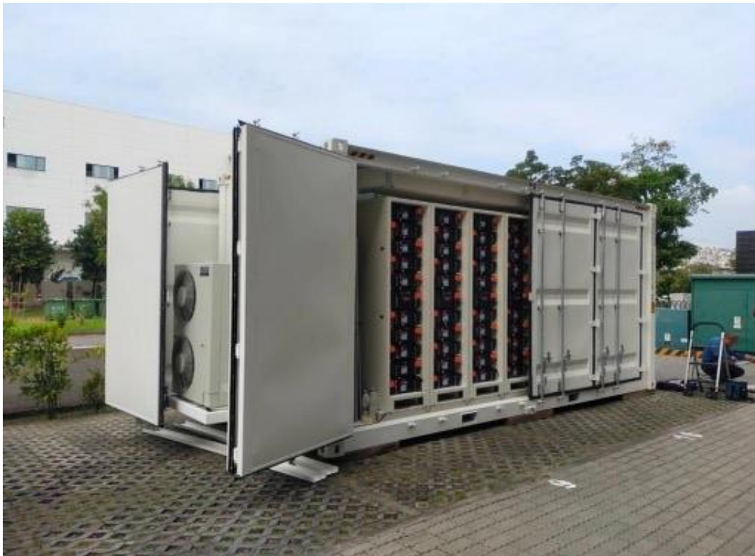
40 foot Containers used for Large Battery Storage Systems, external cooling for climate
