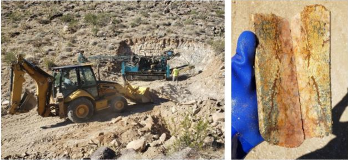
Picture 1&2) After drill rig breakdown, performing additional work to restore the width of the pad for hole MH-08 just before drill suspension decision; Core showing from hole MH-07.
