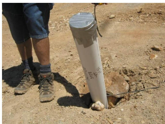
Figure 31. Drill Hole with Temporary Cap.
