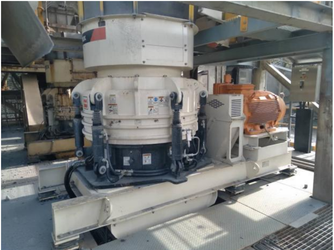
Figure 2: New TC-1000 Crusher Installed and Being Commissioned
