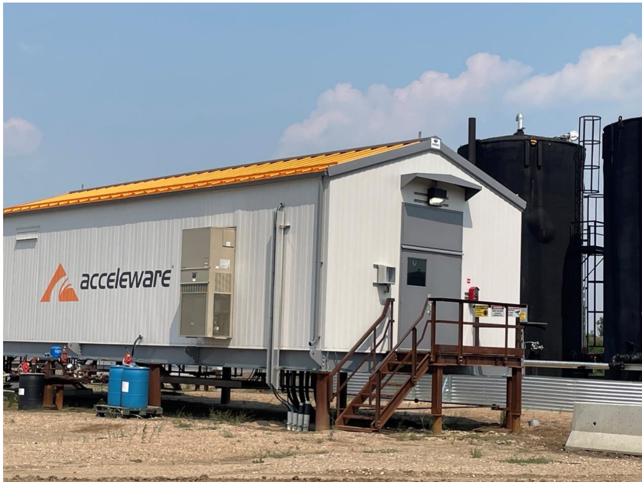
E-house at Acceleware's RF XL Commercial-Scale Pilot Test at Marwayne, AB. July 2023
