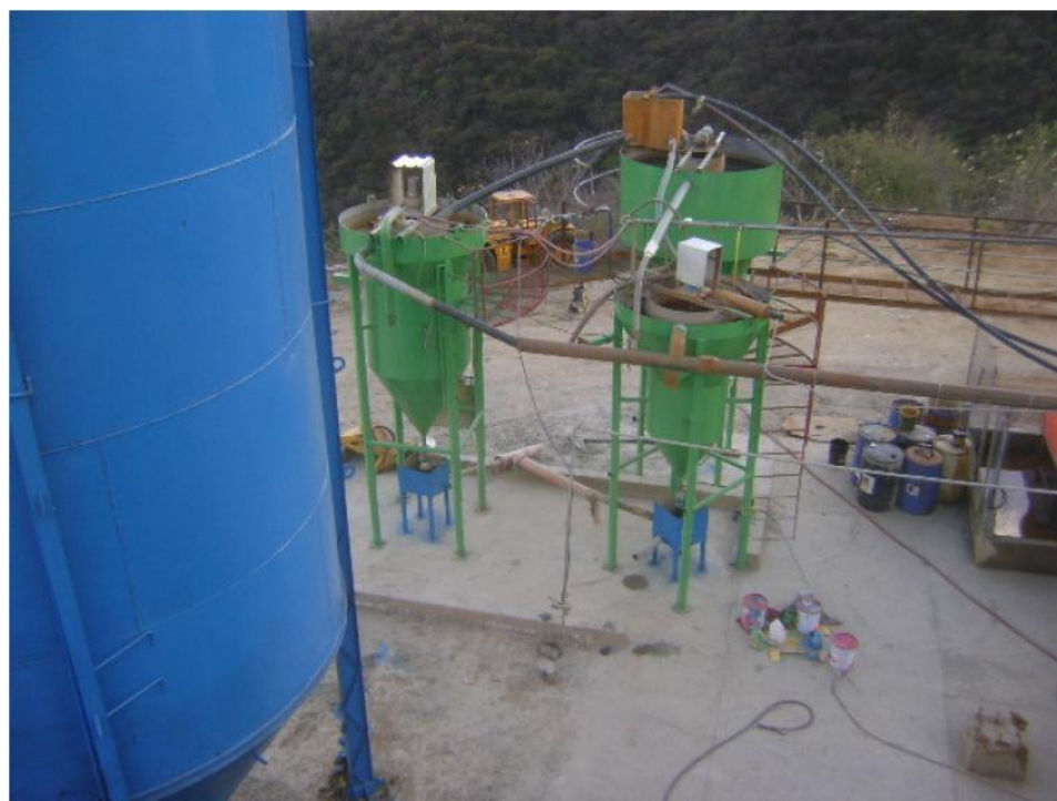
Figure 13.6. Fine Ore Bin and SEDCON final tailings thickeners.
