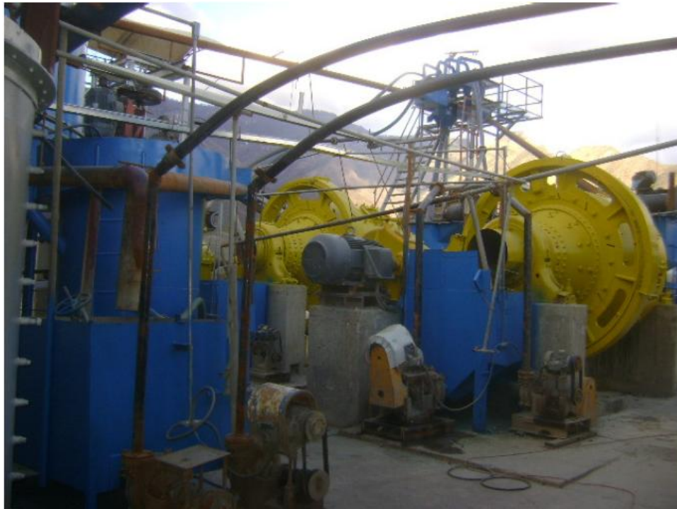
Figure 13.8. From left to right: partial view of the concentrator thickener (gray), tailings sump, scavenging cylindrical flotation cell, ball mill discharge sumps, Hardinge mills and hydrocyclones (behind and up).
