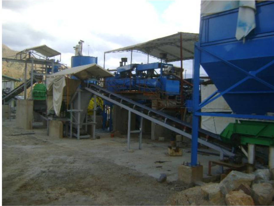
Figure 13.3. From right to left: coarse ore bin (apron feeder in green), belt conveyor No.1, grizzly, jaw crusher, cone crusher, and belt conveyors No. 2 and 3. Also shown is one rougher flotation bank.
