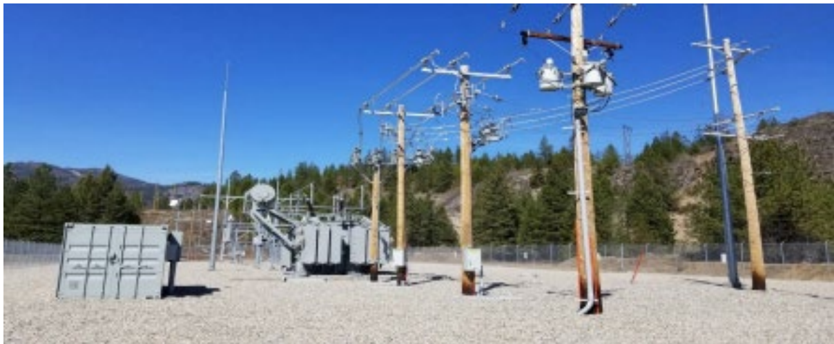
This photo shows a portion of the electrical distribution infrastructure at the Christina Lake Facility.
