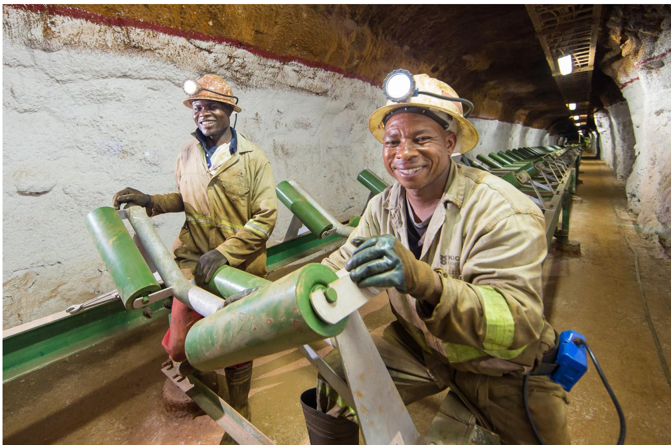
Figure 5: New rollers being installed on the 1,150-metre-level ore conveyor belt as part of the infrastructure upgrading program.
