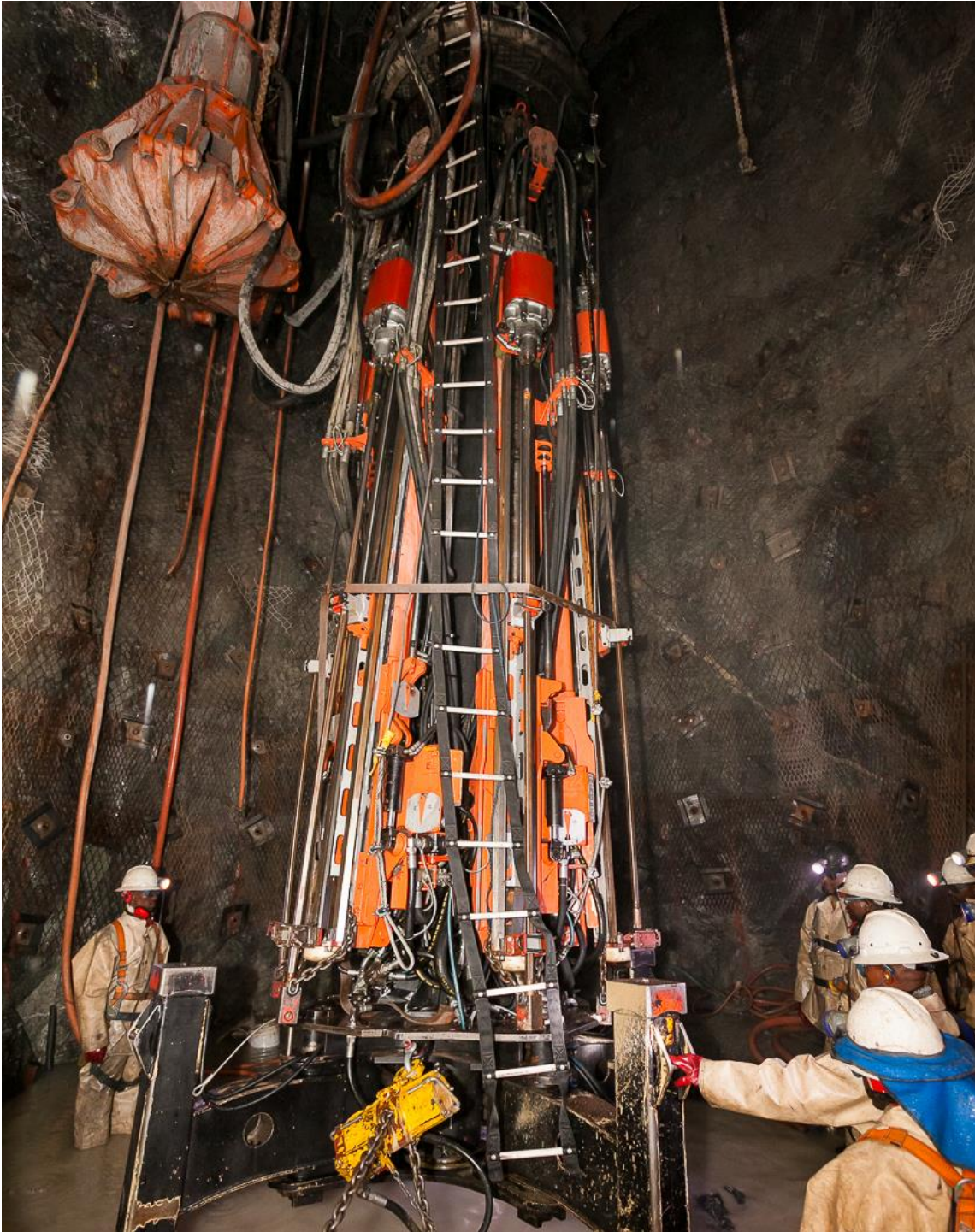
Figure 2: Members of the Platreef sinking team underground in Shaft 1, which was at a depth of 346 metres below surface on May 8, 2017.
