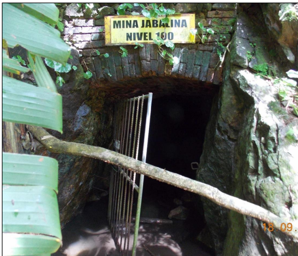
2020 Site Visit. Open steel bar gate at the entrance of La Jabalina drift
