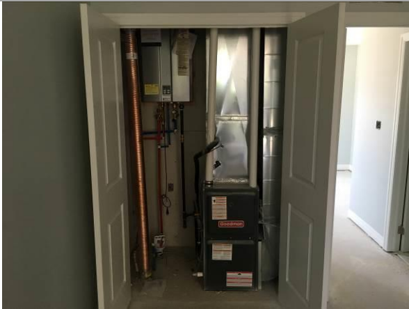
Residence Mechanical Room
