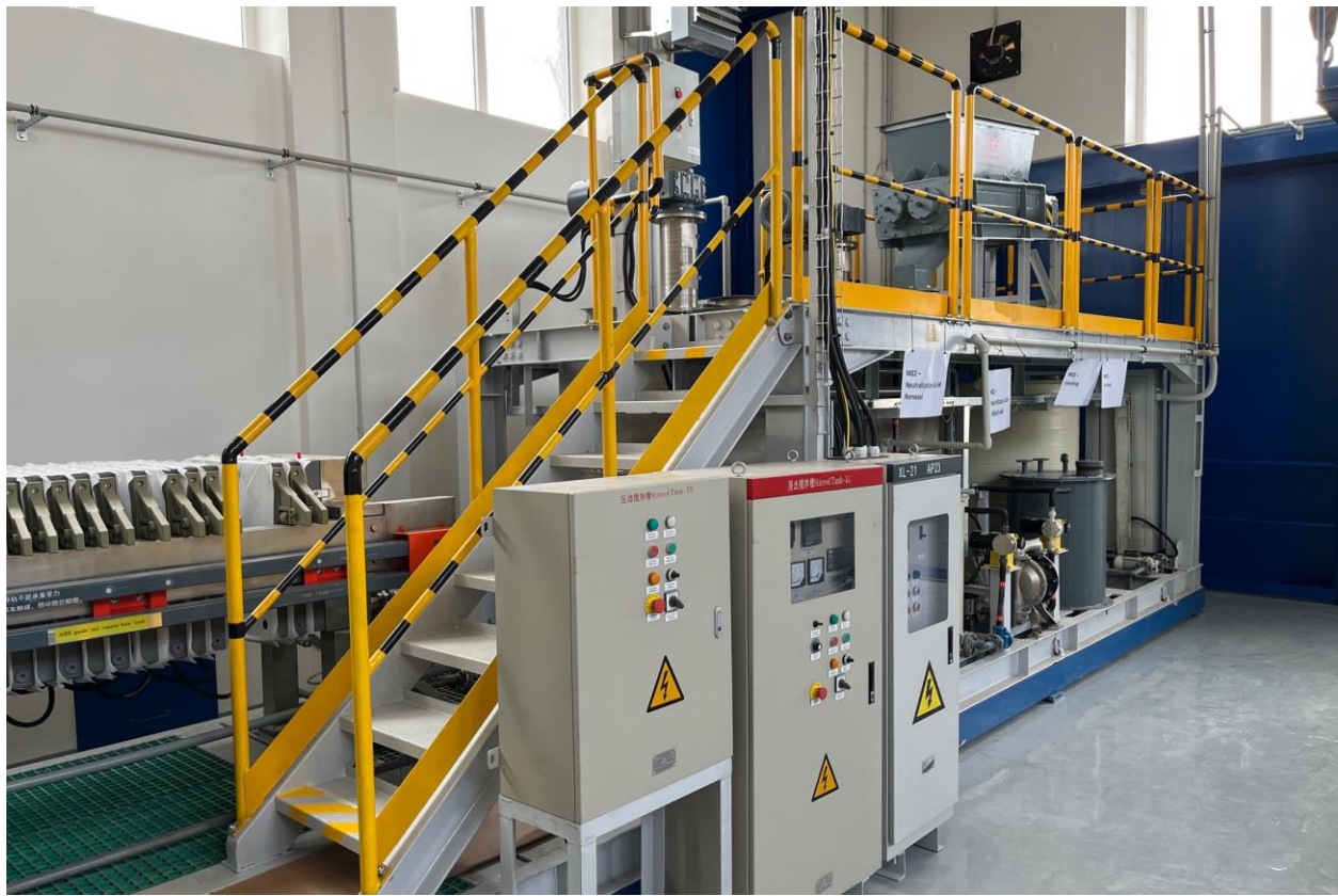
Photo 4. Leaching and Purification Module
