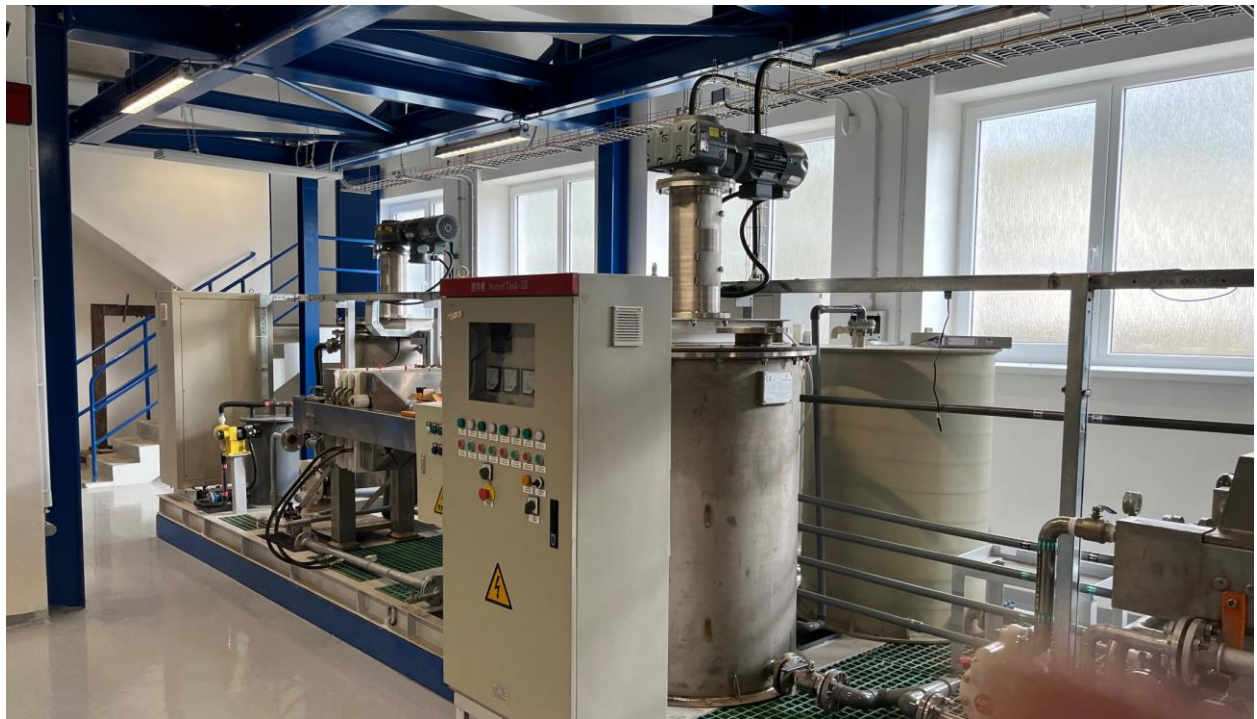
Photo 7. HPEMM Dissolution, Deep Final Purification Module
