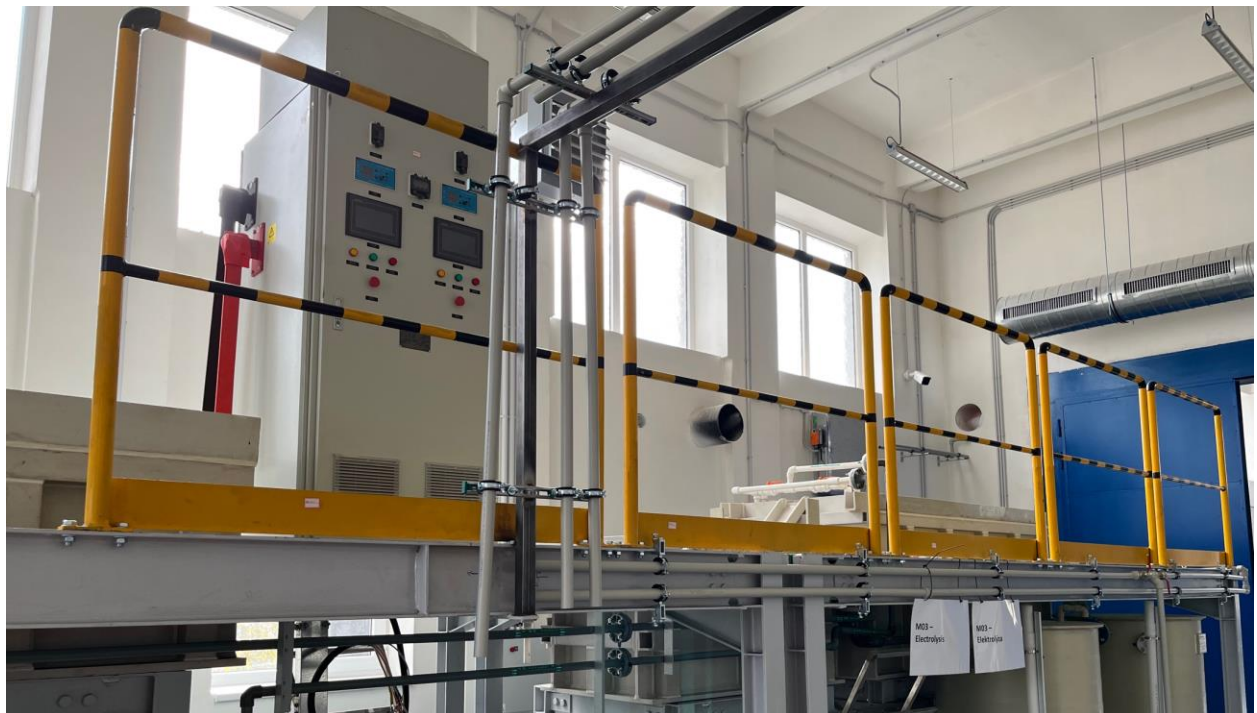
Photo 6. Electrowinning Module (a purification step in its own right)
