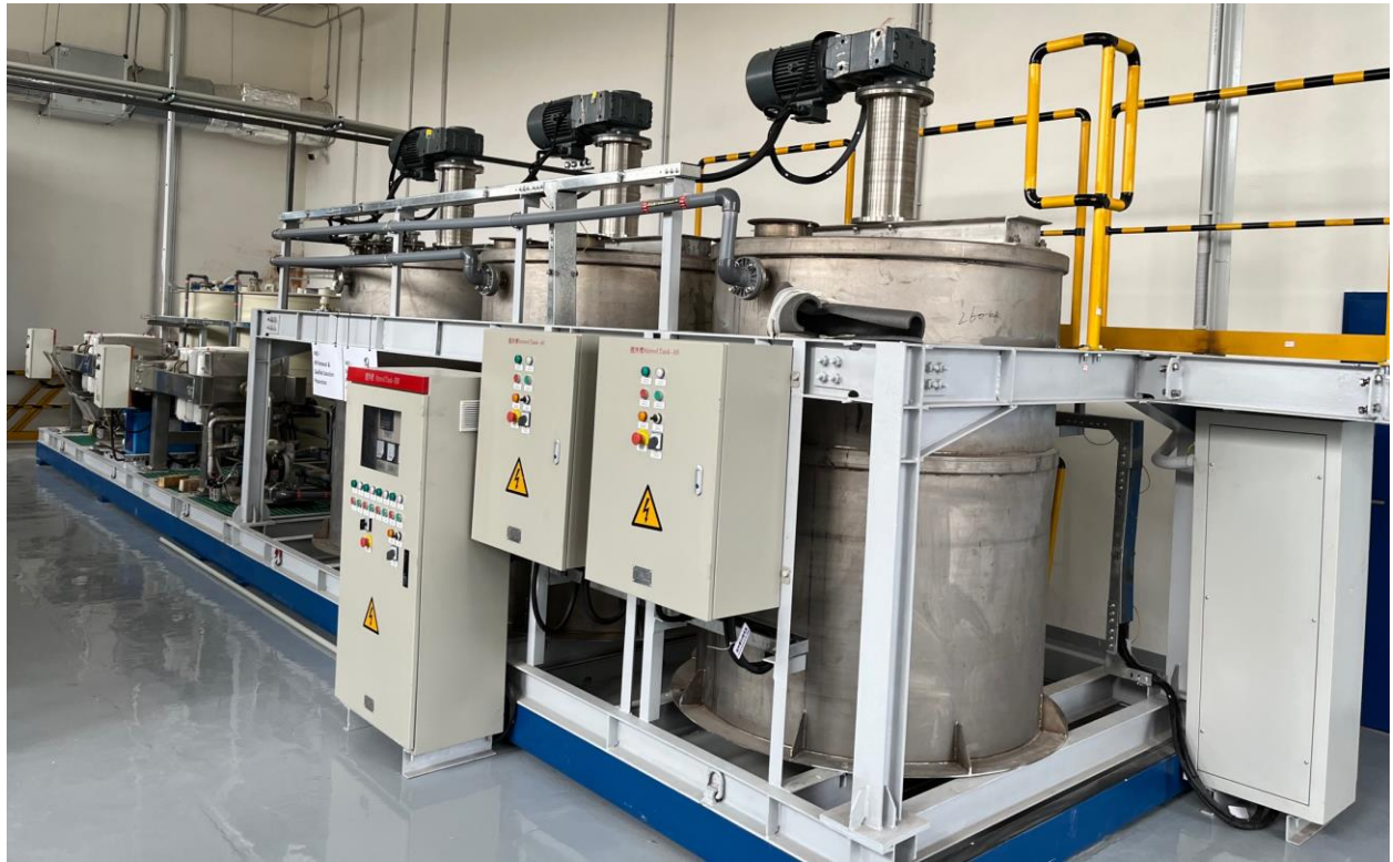
Photo 5. Two Stage Purification Module
