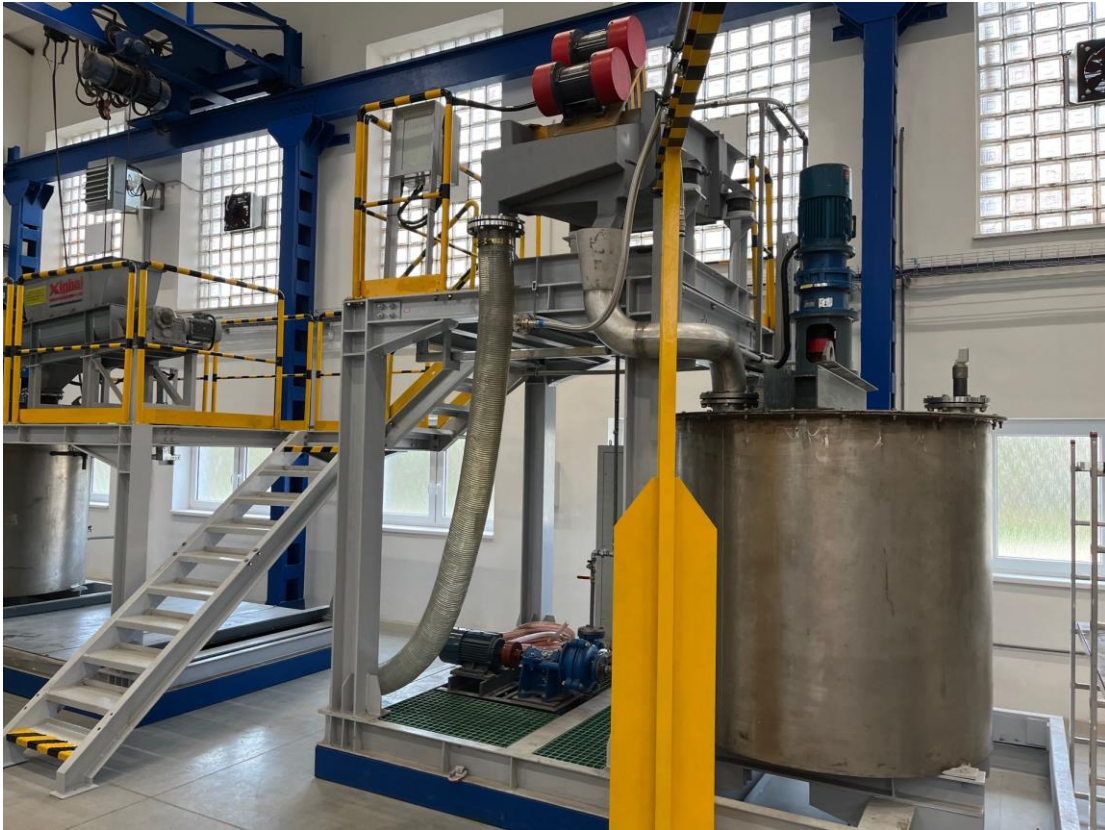
Photo 1. Ore to Slurry Preparation Module
