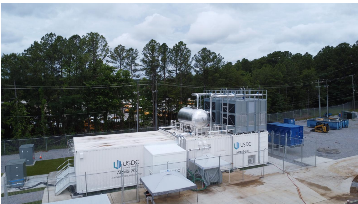
US Data Centers’ ARMS 200 AI-ready modular solution at the Company’s Columbiana, Alabama campus.
