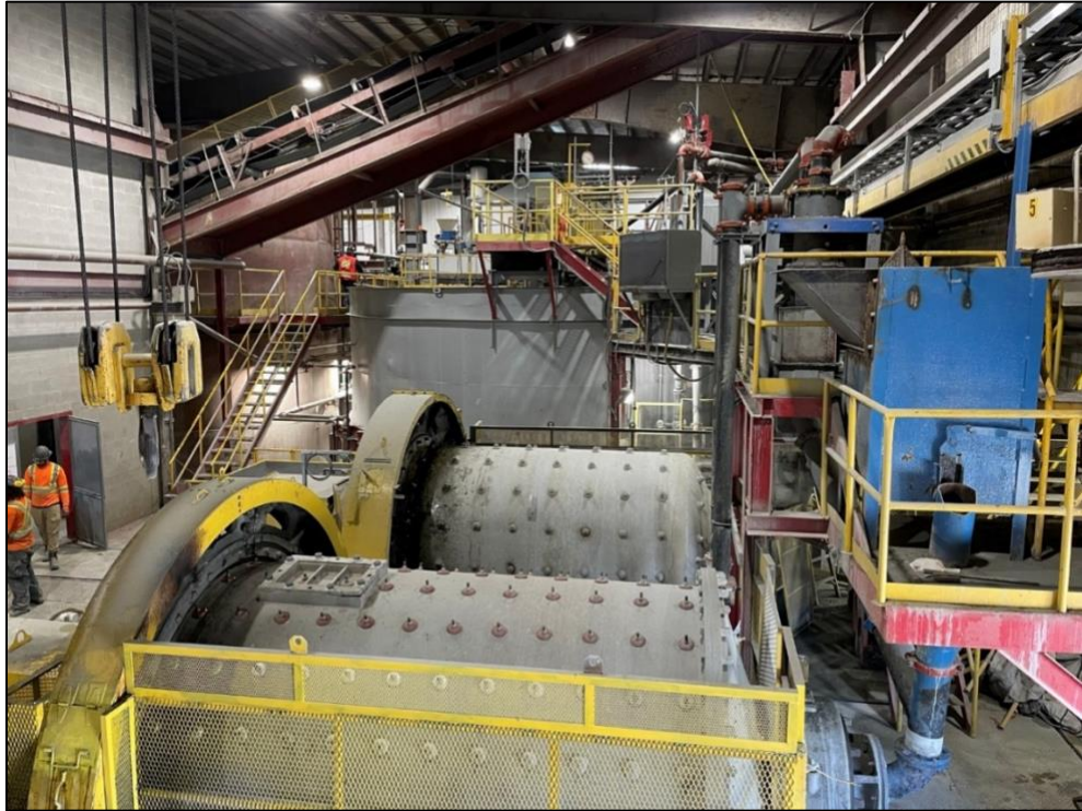
Figure 2: Photo of interior of Beacon Mill currently undergoing detailed inspections for restart
