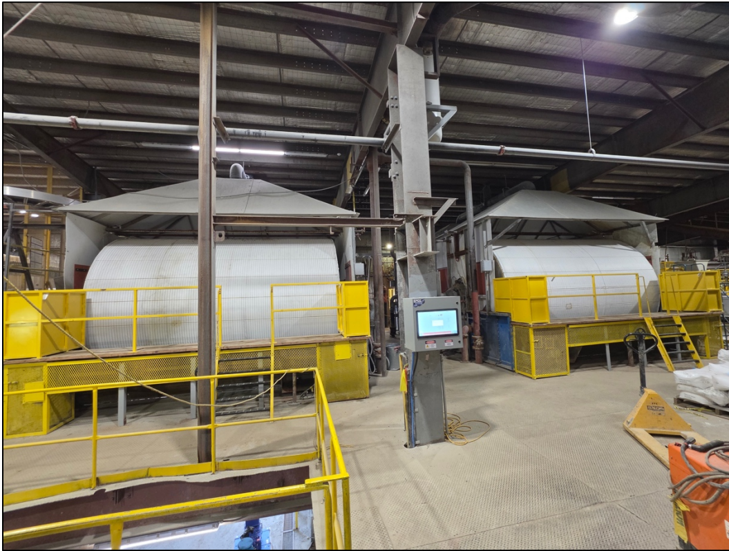
Photo 1: Refurbished rotary drum filtration circuit
