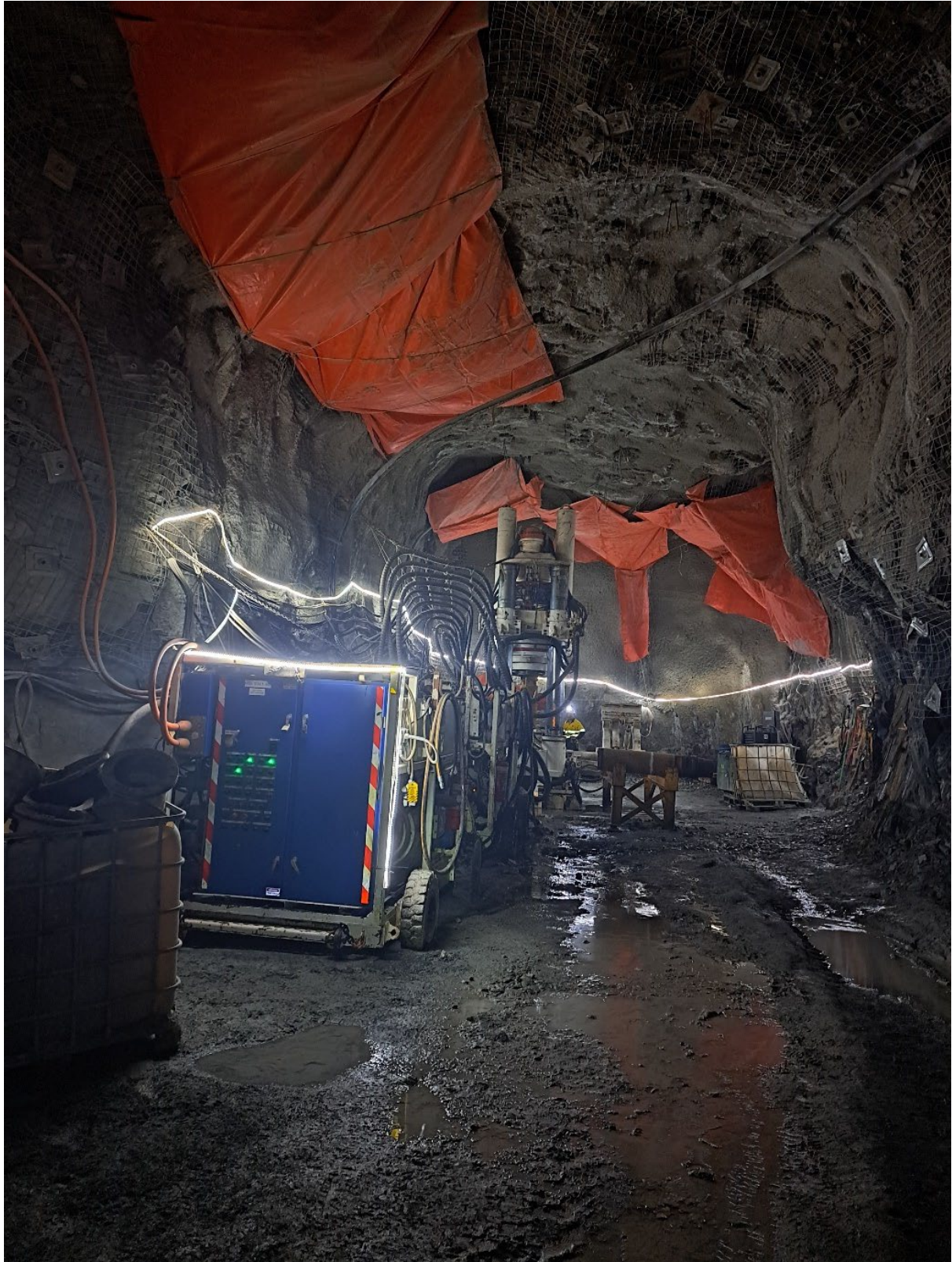
Figure 5 - Long-term ventilation infrastructure under development.
