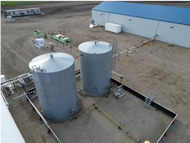
Figure 1 – Project Aurora direct wellhead connected piping for production and disposal brine
