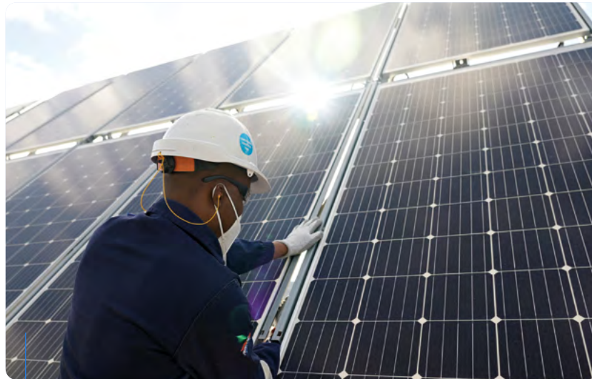
Assembling PV panels for the solar-powered hydrogen plant under construction at our Mogalakwena PGMs mine.
