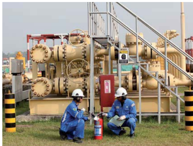
Operations staff carrying out safety checks at the Bangora Field plant, Bangladesh.
