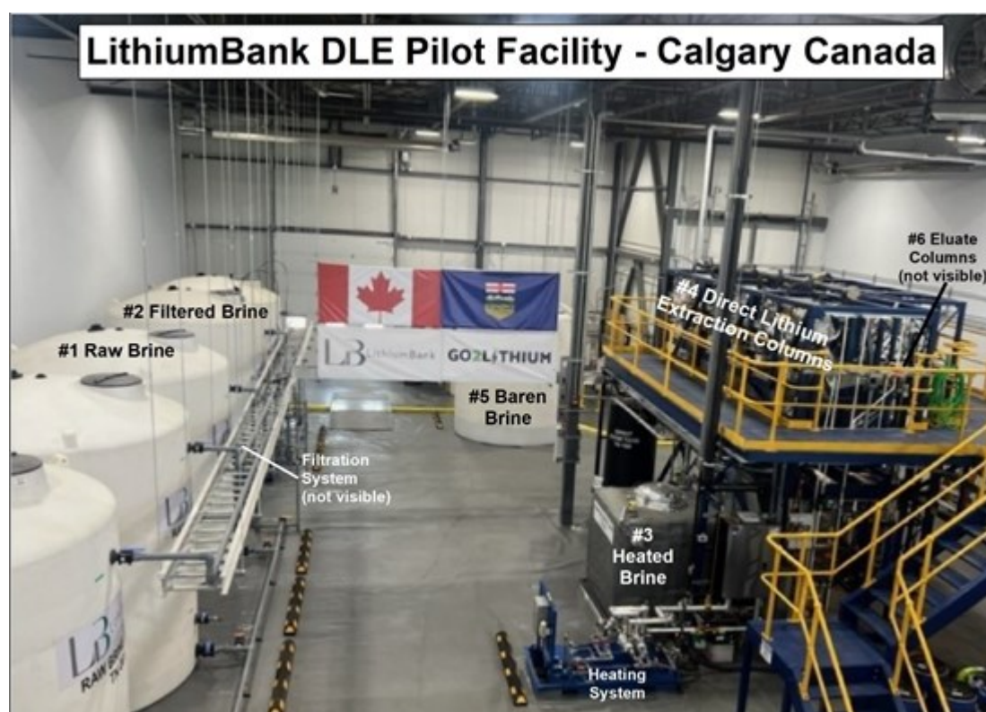
Figure 1. LithiumBank's DLE pilot plant facility: #1 - Raw brine brought in from Boardwalk (raw brine has been through a de-gassing process by AMGAS), #2 - Filtered brine tank holds brine post filtration for suspended solids and hydrocarbons (filtration system not visible in photo), #3 - Heated brine tank is insulated and holds brine at a temperature of ~70°C, #4 - DLE columns continuously move brine and the IX sorbent in a counter current manner, #5 - Baren brine, depleted of lithium is held here until properly disposed of in a disposal well, #6 - IX sorbent was collected for later processing for this particular pilot campaign (not visible in this photo).
