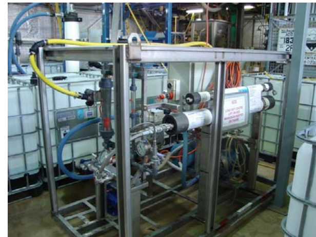
Reverse osmosis and water recycle
