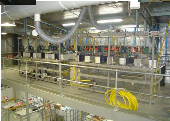
Solvent extraction circuit
