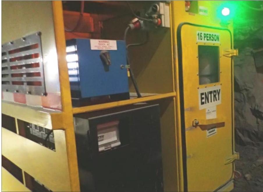
Figure 16-9: Typical underground refuge chamber
